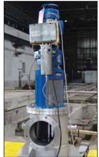
Drive unit on top of an evaporator
