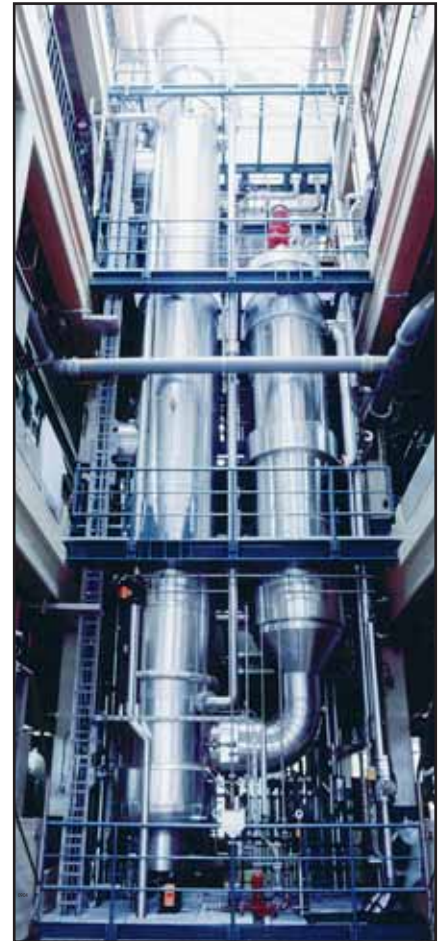
Rectification plant with thin film evaporator for solvent regeneration
