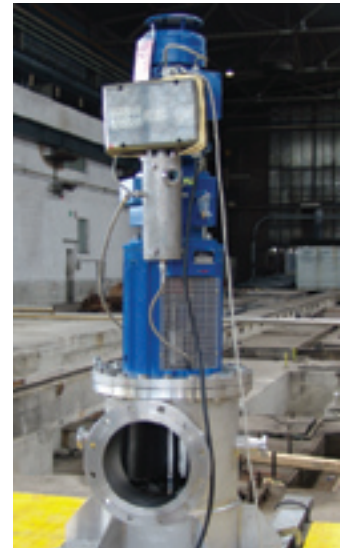
Drive unit on top of an evaporator
