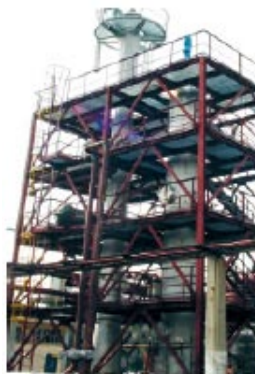
Fig. 1. Extraction plant Rompetrol Vega Refinery, Ploiesti/Romania.
